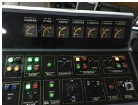
Fig. 5. Panel of Monitors and Controllers
