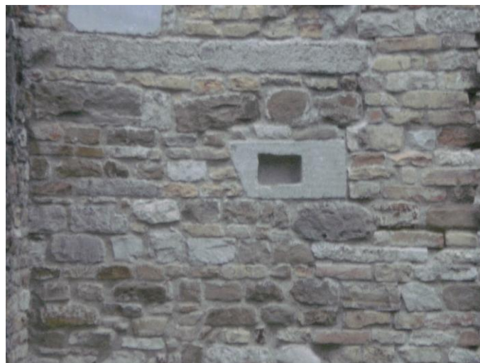
Fig. 6. Rectangular base from the theatre in the W wall of the Baptistery (the Author, 2012).
