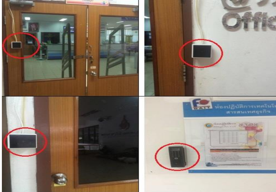
Fig2. An RFID setting in front of rooms from the testing site
