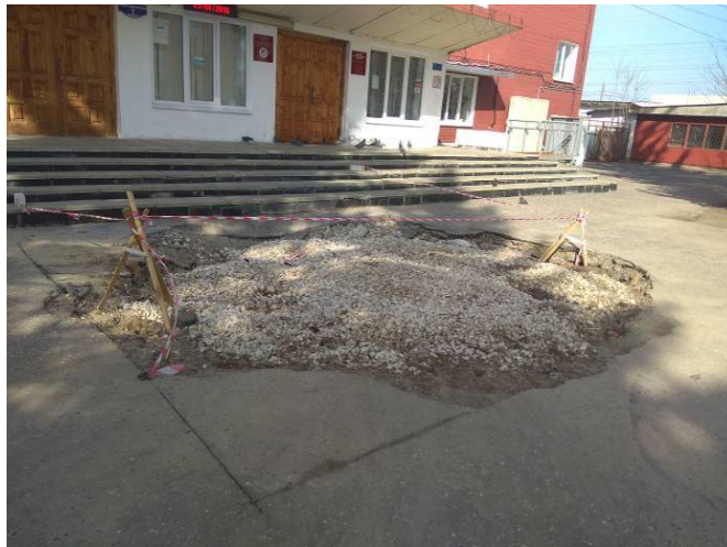
Fig. 5. The resulting failure at the site of the development of suffusion. Source: (Dorofeev, Kuzichkin, Grecheneva & Baknin, 2018).
