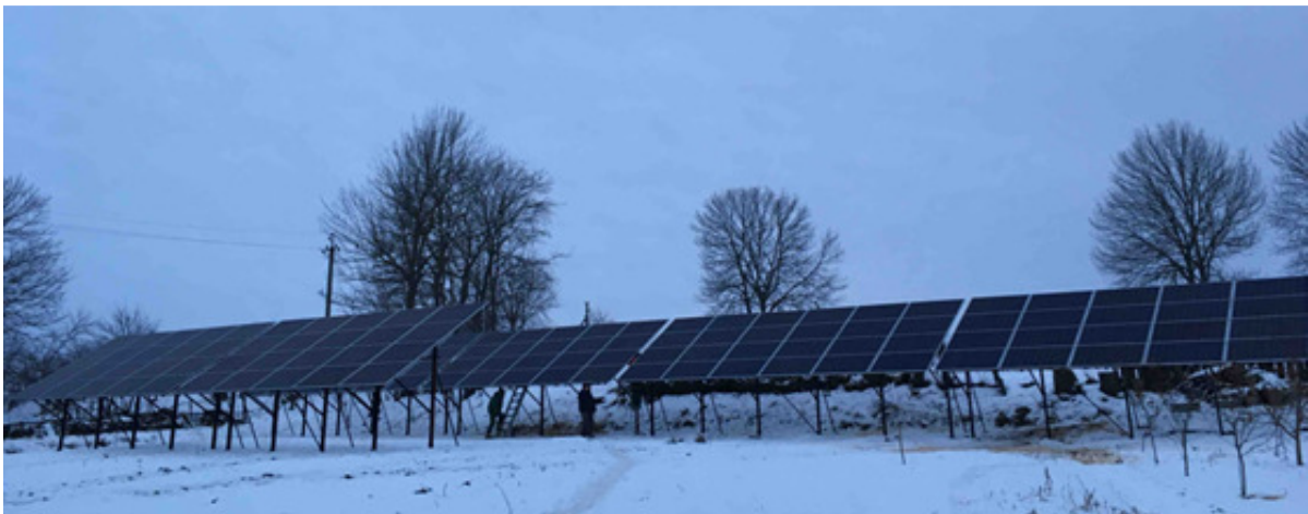
Figure 1: Photo of the solar power plant in Zelene village
