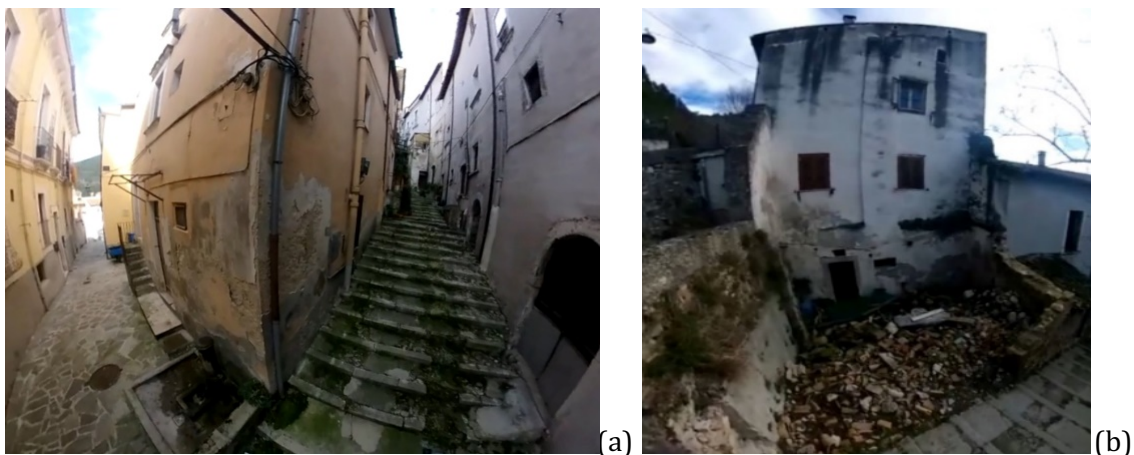
Figure 6: View of the alleys in the historic center in poor maintenance condition (a) and cracking pattern with collapse (b) of buildings in Popoli Terme (PE).
