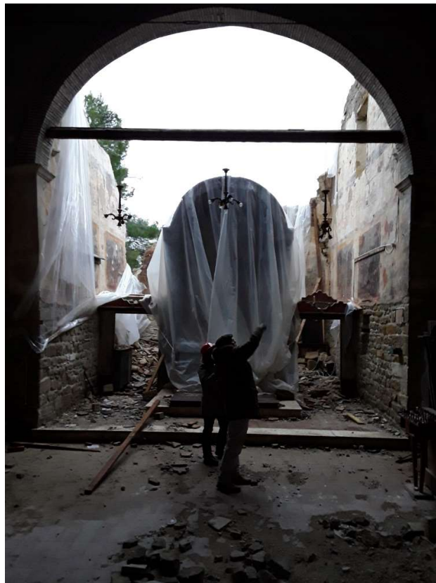
Figure 3: Interior of the Sanctuary of Madonna di Garufo (Sanctuary), damaged by the 2016 earthquakes. Source: ICCD, Usage Terms: Cultural Heritage Standards (BCS).
