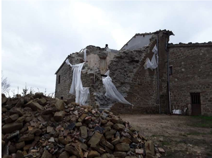
Figure 2: Exterior of the Sanctuary of Madonna di Garufo (Sanctuary) after the 2016 earthquake in Camporotondo di Fiastrone (MC). Source: ICCD, Usage Terms: Cultural Heritage Standards (BCS).
