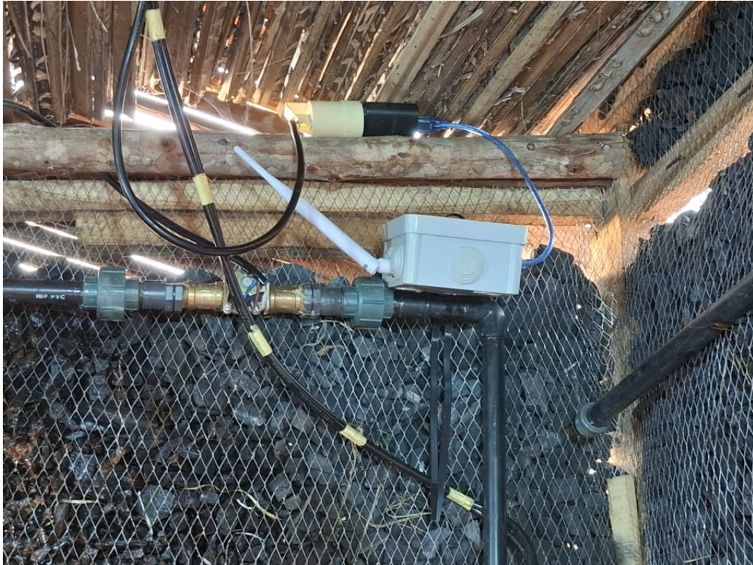
Figure 4: Prototype deployed on-site in Saketé: ADXL345 sensor fixed on the pipeline
